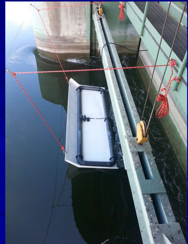
Installed 10' floating antenna in west spill bay March 31, 2015
